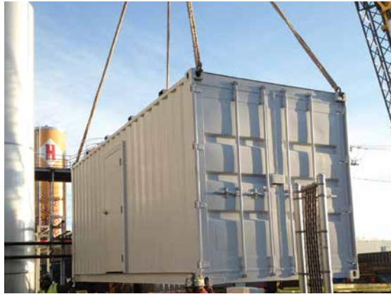
In 2013, Harpoon Brewery installed a co-generation system at their Boston Brewery to simultaneously generate electricity and heat.
