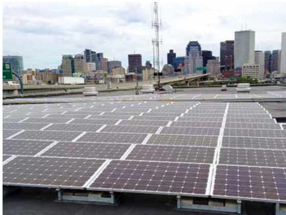
In 2012, the City of Boston installed solar panel arrays on the roof of the City Public Works Facility to apply green technologies to power the emergency operation of traffic control systems at 18 intersections along the City of Boston’s evacuation route.
